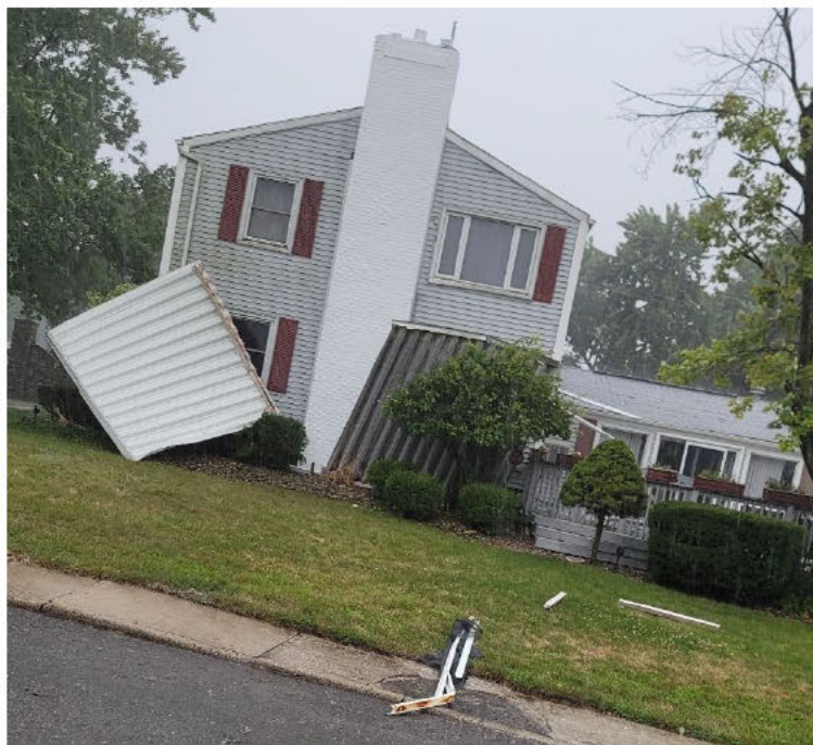
The disaster: the structure was torn off by storms and a significant portion landed on 3 Melrose Manor.
