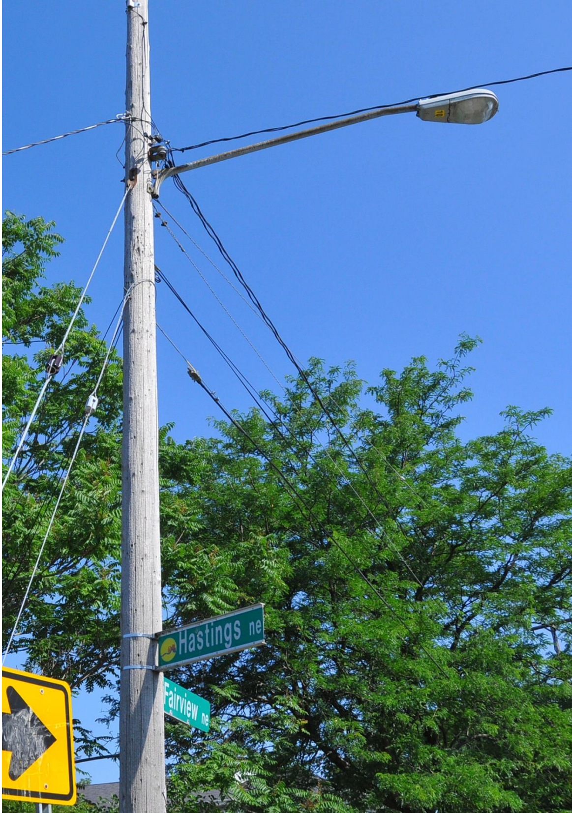
P1 Wood Pole with Cobra Head Luminaire
