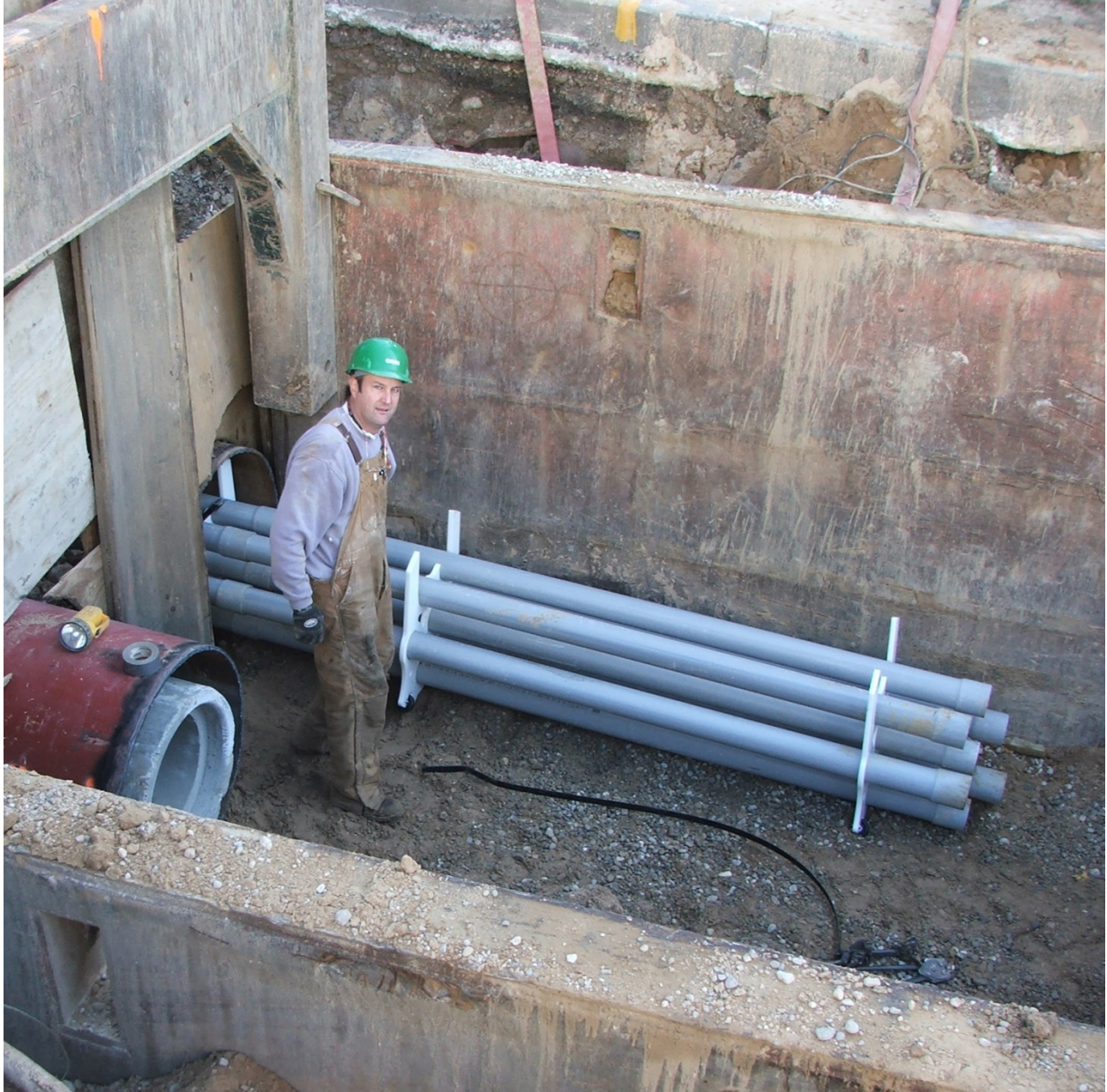
P5 Duct alongside Storm Sewer under US131
