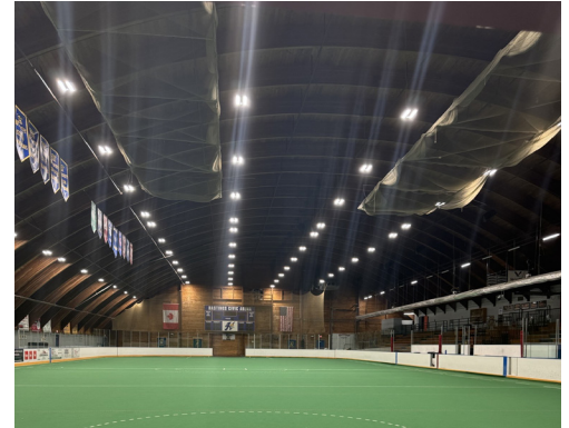
Pictured (above) rooftop solar panels, (below) new LED lighting.
