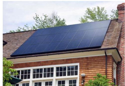
Figure 4. Roof-mounted solar panels
