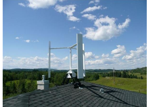
Figure 3. Roof-mounted wind energy system
