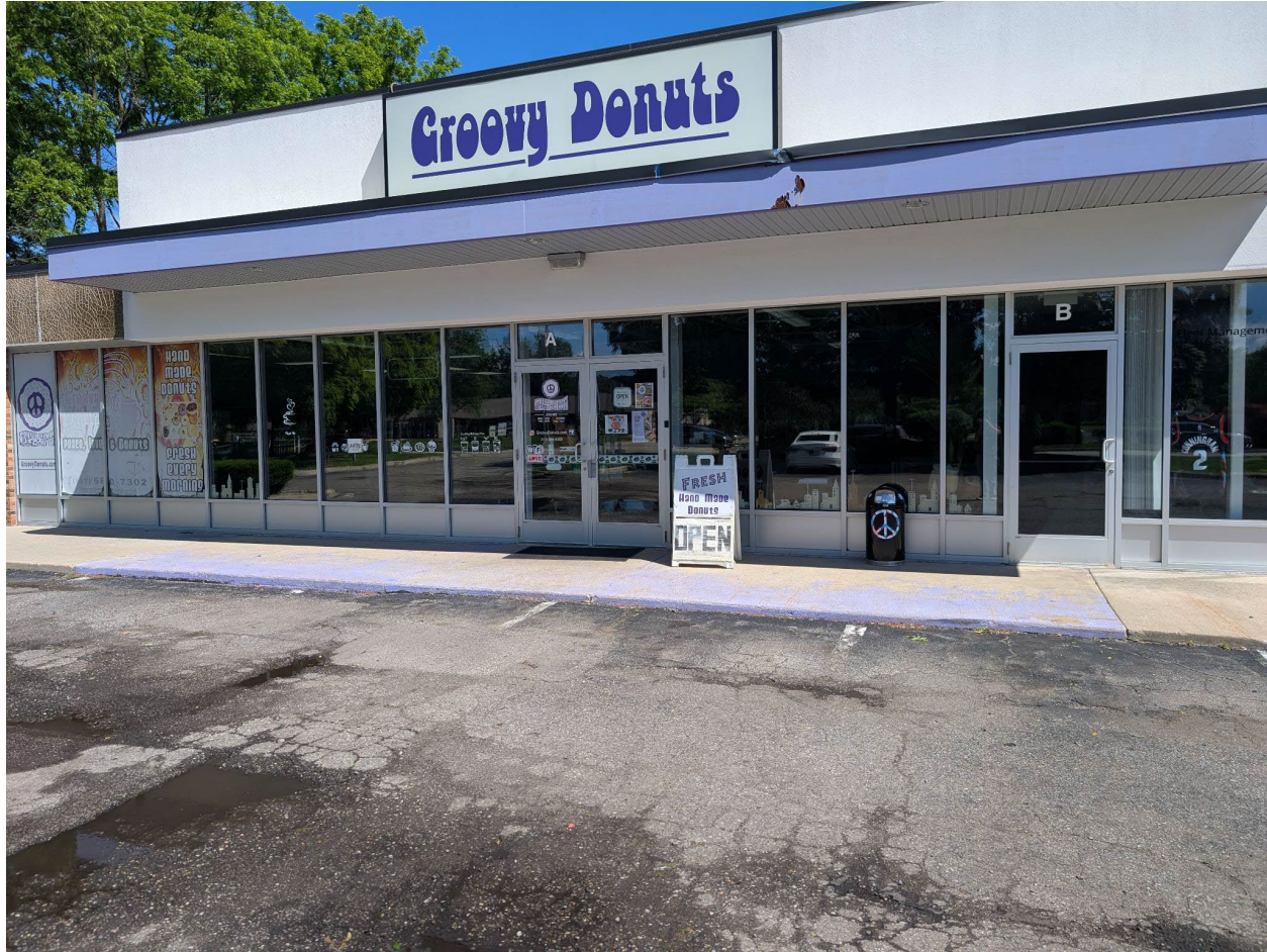
Wide view of the existing front parking area showing extensive alligator cracking, surface deterioration, and blue chalk markings laying out the proposed location of the new ADA-accessible parking space and access aisle in front of the Groovy Donuts storefront entrance.
