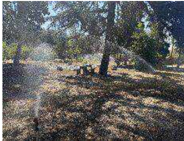
Installed irrigation system operating within the restored project area.
